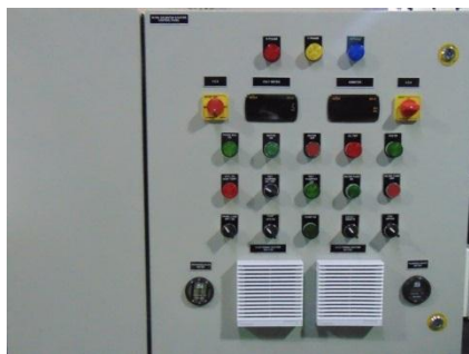
Electrical Pump Panel 45, 75, 90, 120 KW
